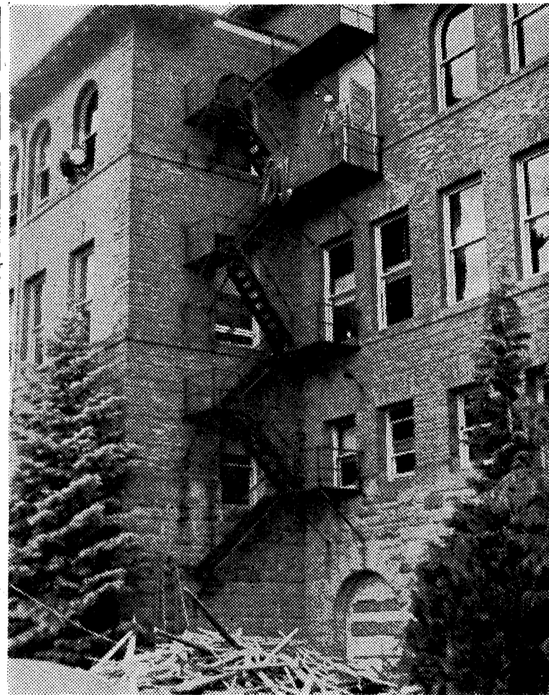
OUT THE WINDOW—A workman on the second-floor fire escape hurls another portion of the dismantled old auditorium onto the pile on the parking lot. The old balcony has been completely removed. The space is being converted into classrooms which will be ready for use this fall quarter.—Justin Nix photo.
