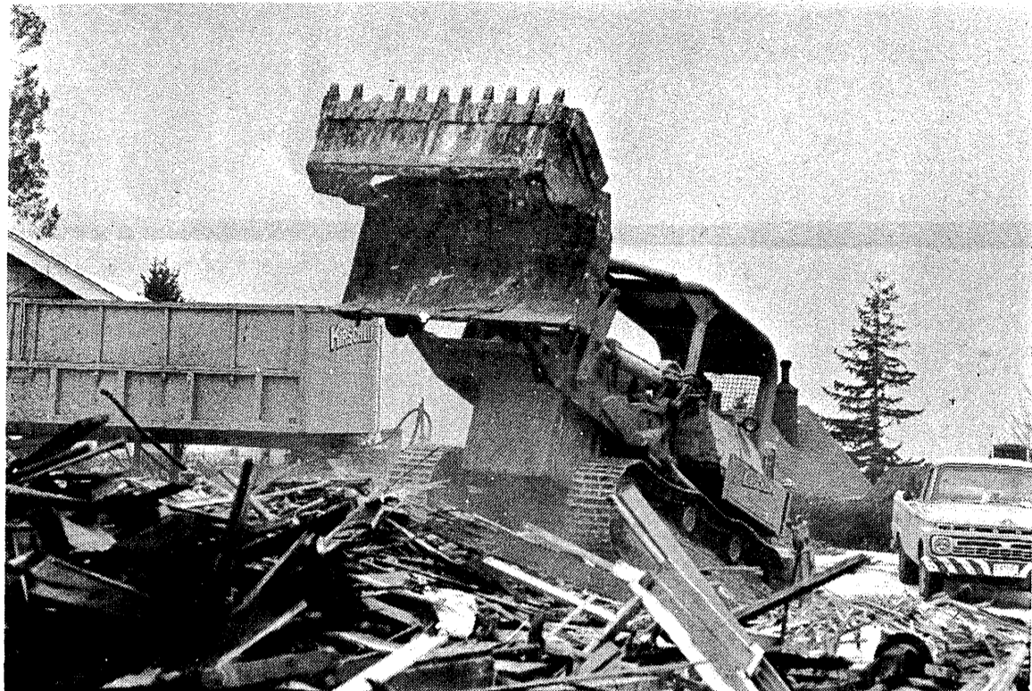
MECHANICAL MONSTERS put a quick end to another old campus landmark last week as construction crews hustled to complete several major projects. Photo by BILL WOODLAND
