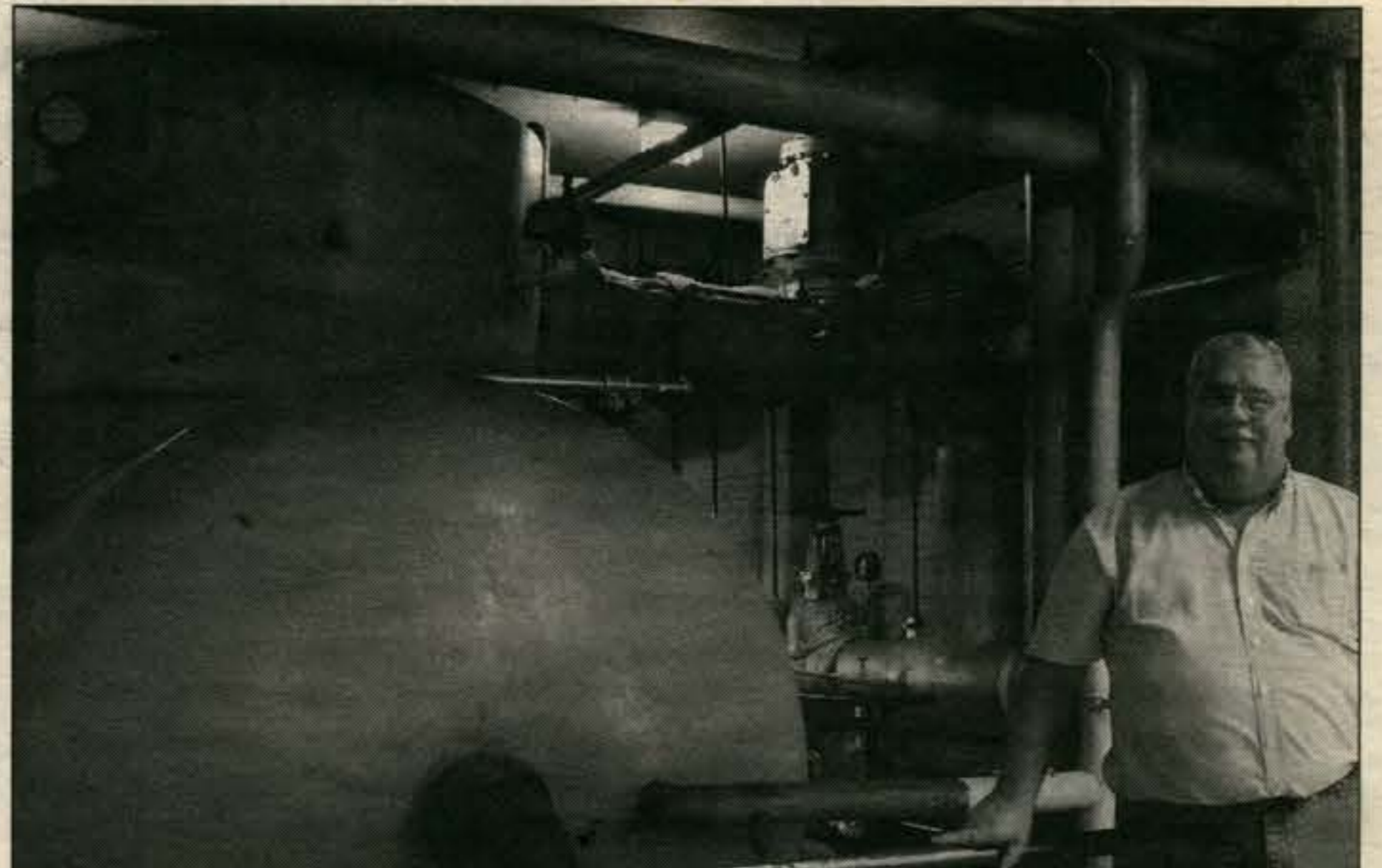
Paul Hughes, chief engineer of Western's Steam Plant, poses amid an array of pipes inside the Steam Plant on Monday.
