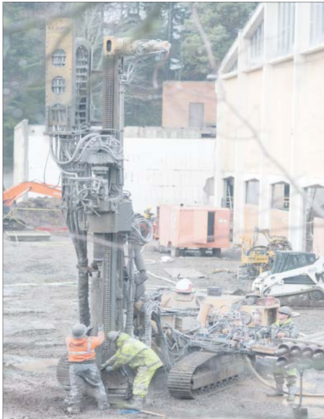
Construction crews working on Sam Carver Gymnasium on Tuesday, Jan. 5, drill ground supports deep into the earth to prepare for further construction on the new building. // Photo by Ian Koppe
