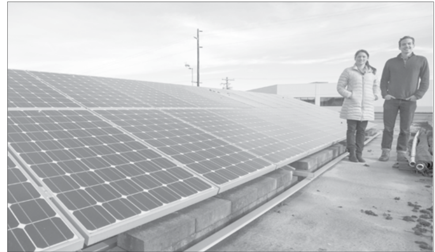
Rose Lathrop, the Green Building and Smart Growth Program Manager at Sustainable Connections, and Western senior David Jackman, the Energy Program Assistant, stand next to the solar panels installed atop the Sustainable Connections building on Ellis Street on Wednesday, Jan. 6. The project they are working on will donate panels to the Bellingham Food Bank later this year. // Photo by Western Front staff
