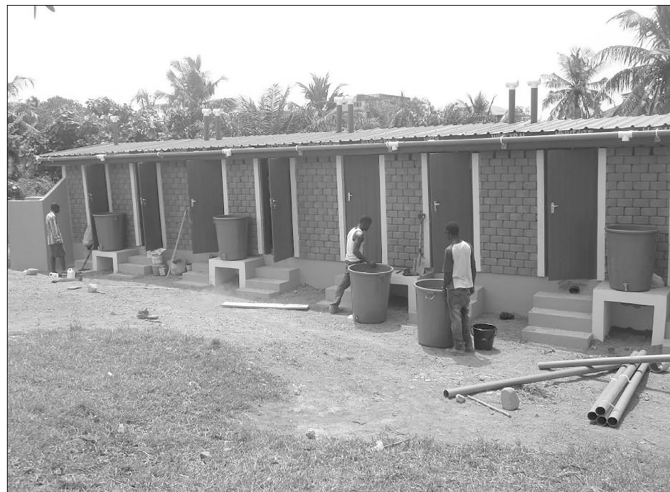
Compost-latrine project designed by the Northwest chapter of EWB-USA in Ghana in 2009. // Photo courtesy of Colleen Mitchell
