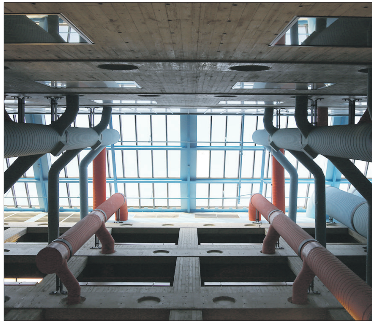
Looking up toward the skylight inside the Environmental Studies building on Monday. // Photo by Mathew Roland
