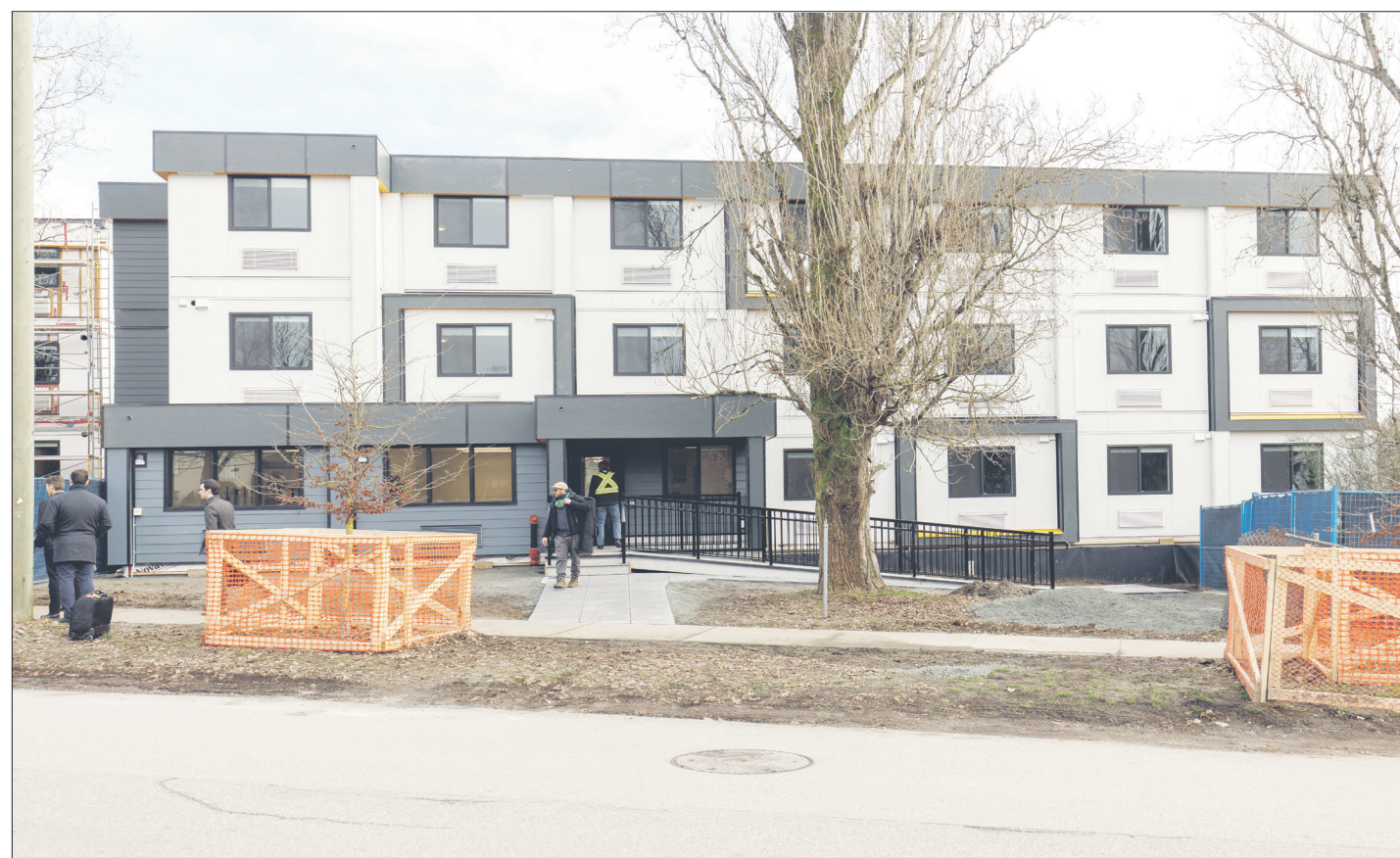
Construction nears the end on a BC Housing low-income residence. // Photo courtesy of BC Housing
