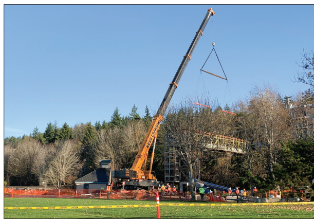
A construction crew works to dismantle Boulevard Park's pedestrian overpass on Nov. 21. // Photo by Noah Harper
