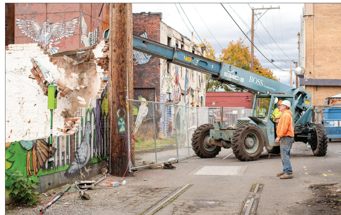
A portion of Bird Alley is demolished on Oct. 16. due to fire damage from the fire at Hohl Feed & Seed. // Photo by Max Gleiberman
