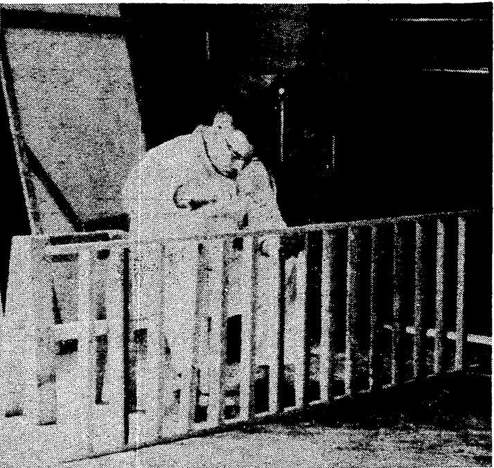
This special feature shows some of the construction work that is going into the set for next week's production or "Shenandoah." Twelve people have been working for three weeks preparing the three full sets necessary for the show. Paul Waldo is the technical set director. (Photos by Cal Cole, Collegian photographer.)
